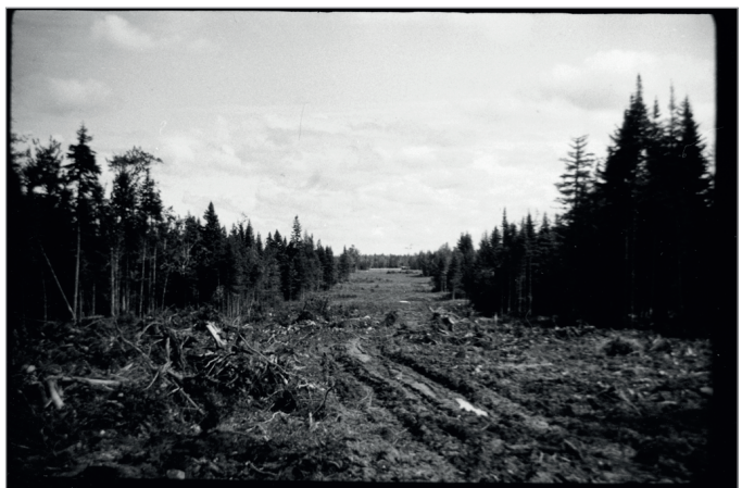
FIG. 6. CMHC ENGINEERING CREWS CLEARING ROAD CORRIDORS THROUGH THE THICK BUSH IN THE OROMOCTO TOWNSITE, 1954-1955. MAJOR ROADS WERE SEPARATED FROM ADJACENT HOUSING BY UNCLEARED BANDS OF FOREST. | CMHC PHOTO 1101-1124-013.
