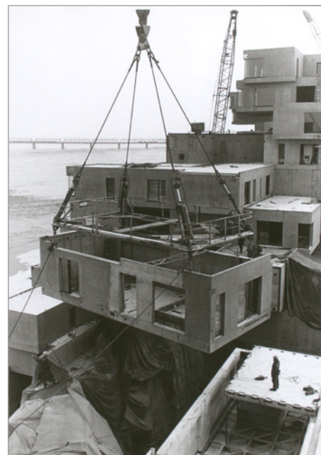
FIG. 19. GANTRY CRANE LIFTING MODULE INTO PLACE, 1966-1967. | SAFDIE ARCHITECTS. SOURCE: MOSHE SAFDIE FONDS, CANADIAN ARCHITECTURE COLLECTION, MCGILL UNIVERSITY LIBRARY, MONTREAL. COURTESY: SAFDIE ARCHITECTS.
