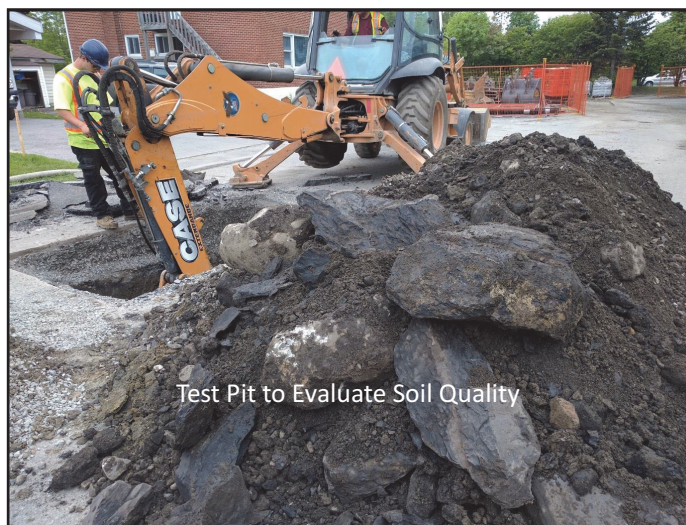
Figure 4. Example of test pit excavation to assess soil quality in the area of infrastructure renewal in Case Study #3.
