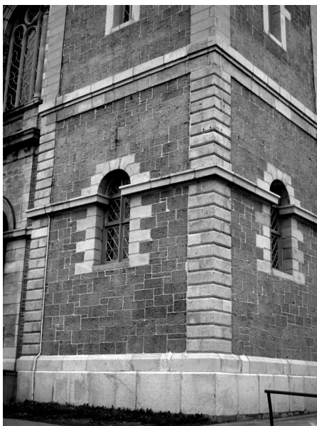
Figure 6 View of the east tower of the Basilica, bases and quoins constructed with Leinster granite and rubble facing with Gibbett Hill sandstone.
