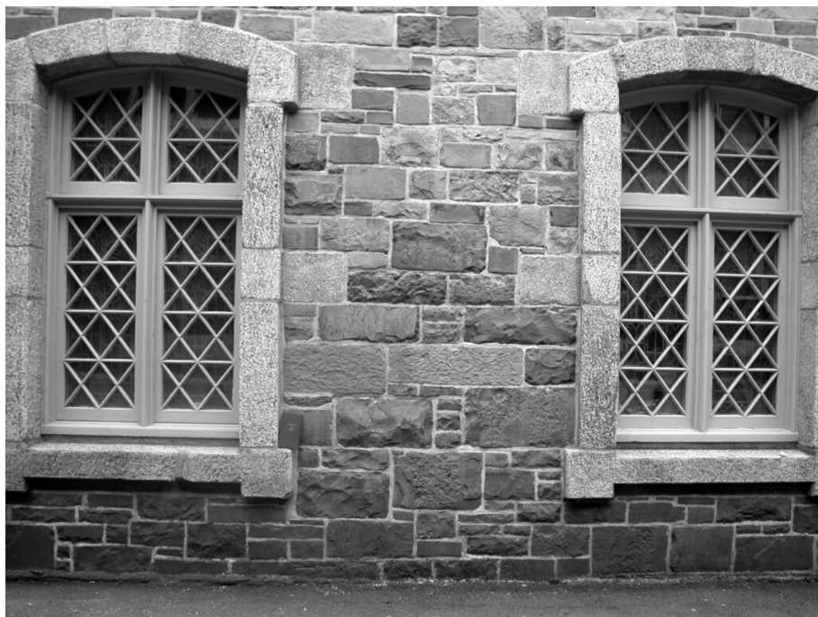
Figure 10 View of the west ambulatory wall. Blocks of fossiliferous light grey Galway limestone are surrounded by sandstone blocks from Kellys Island, Mistaken Point, and Gibbett Hill, with Leinster granite dressings around the windows.
