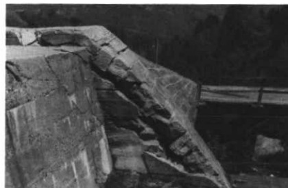
Figure 8 Wing of a check-dam, being slowly crushed by lateral pressure resulting from deepseated creep along unstable flanks of a torrent channel near Crodo, Italy.
