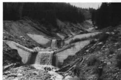
Figure 7 New check-dams along a deeply scoured source area of residual colluvium near Inzing, Austria. These dams, arranged in a stacked pattern, confine the torrent to a central line and create a more balanced profile, thus preventing erosional instabilities along the embankments. Note the gently rising stone carapaces on either side of the discharge section of the check-dams; they are designed to accommodate the passage of small debris flows without endangering the lateral abutments.
