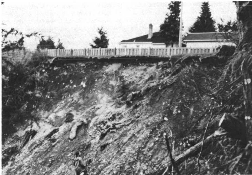
Figure 12 Shallow failure of surficial debris along a steep terrace rim along the eastern coast of Vancouver Island. Failure occurred during an intense rainstorm in December 1979.
