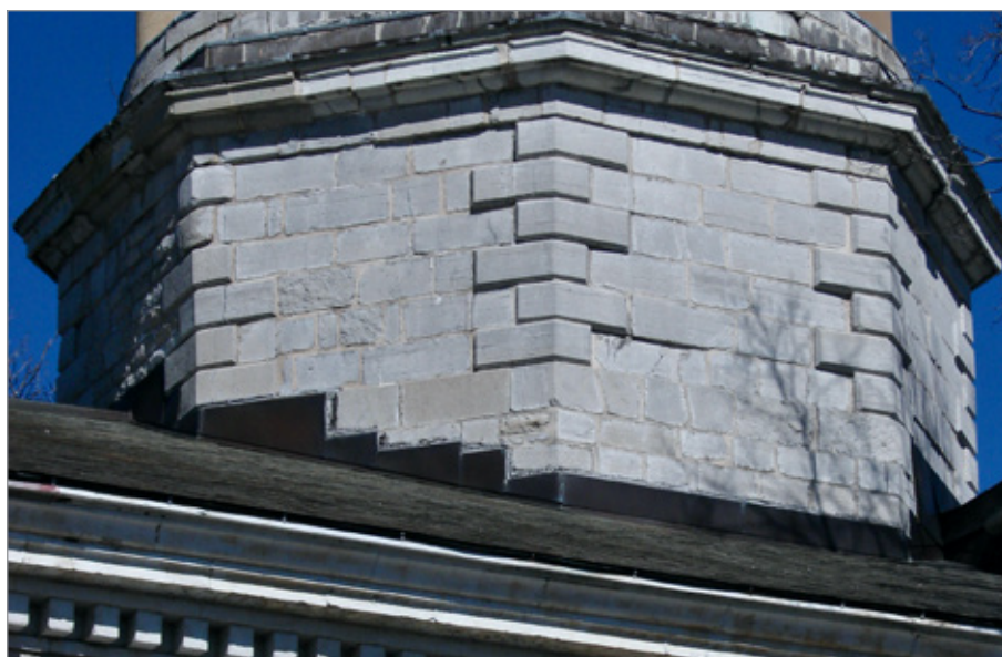
FIG. 16. ST. GEORGE'S ANGLICAN CHURCH, OCTAGONAL BASE OF TOWER, 1841-1842. | PHOTO: PAUL CHRISTIANSON, MAY 2022.
