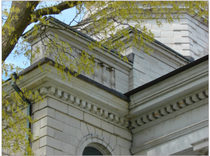
FIG. 45. ST. GEORGE'S CHURCH, PORTICO AND RITUAL WEST FAÇADE, 1842; DETAIL OF ENTABLATURE AND PARAPETS. | PHOTO: PAUL CHRISTIANSON, JANUARY 2020.
