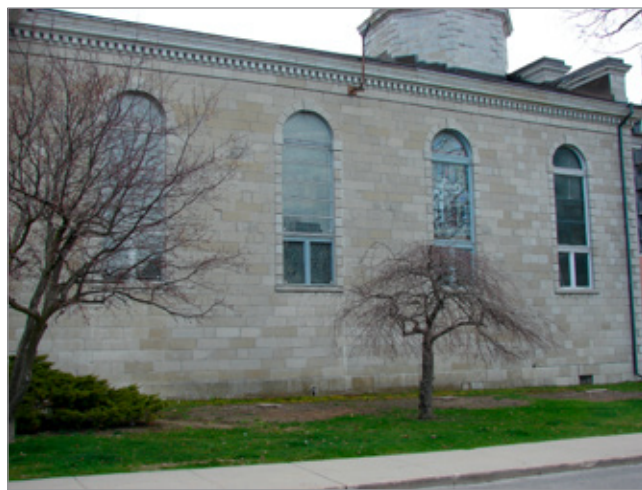
FIG. 4. ST. GEORGE'S CATHEDRAL, KINGSTON, ONTARIO, RITUAL SOUTH FAÇADE. DETAIL OF THREE BAYS FROM 1825-1826 AND ONE BAY FROM 1839-1841, ALL AS MODIFIED IN 1891. | PHOTO: PAUL CHRISTIANSON, APRIL 2020.
