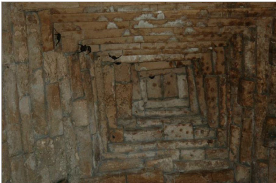
FIG. 15. INTERIOR OF THE ŚIKHARA OF THE LATE SIXTH-CENTURY SŪRYA TEMPLE, NEAR GŌP IN GUJARAT, INDIA. | LIBBIE MILLS, DECEMBER 2010.
