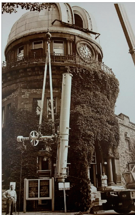
FIG. 10. FIFTEEN-INCH DOMINION TELESCOPE HOISTED FROM THE DOME OF THE DOMINION OBSERVATORY FOR TRANSFER TO CANADIAN SCIENCE AND TECHNOLOGY MUSEUM (CSTM), 1974. | DOMINION OBSERVATORY FONDS, BOX #2, CANADA MUSEUM OF SCIENCE AND TECHNOLOGY ARCHIVES, OTTAWA, CANADA.
