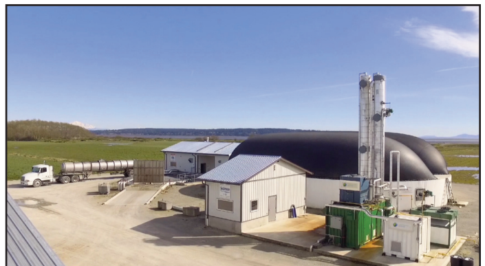
Seabreeze Farm Renewable Natural Gas plant, Delta, British Columbia (Photo: Greenlane Biogas).
